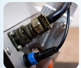
Armoured cable connectivity
